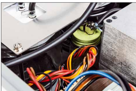
Here you can see filters for moisture separation in the air treatment system
